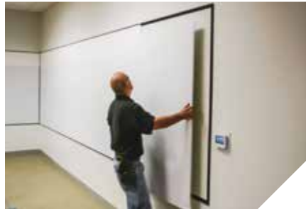
Acoustic Insulation Infill
