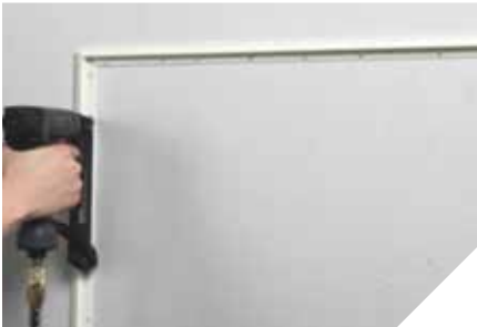
PVC profile framing on wall
